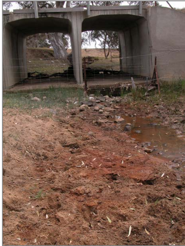
Figure 6.2 Iron Staining at Naringhil Creek Left behind from evaporated groundwater (Site N3) in October.
